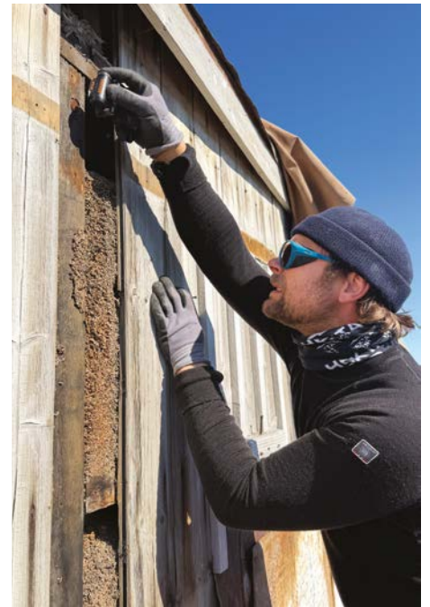
Heritage Carpenter Martin Herrmann investigates the building at Shackleton's Nimrod hut. © AHT/Zack Bennett
